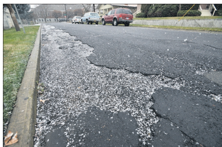
The asphalt is degrading and pitting out along a stretch of Bailey Avenue in Pendleton.
