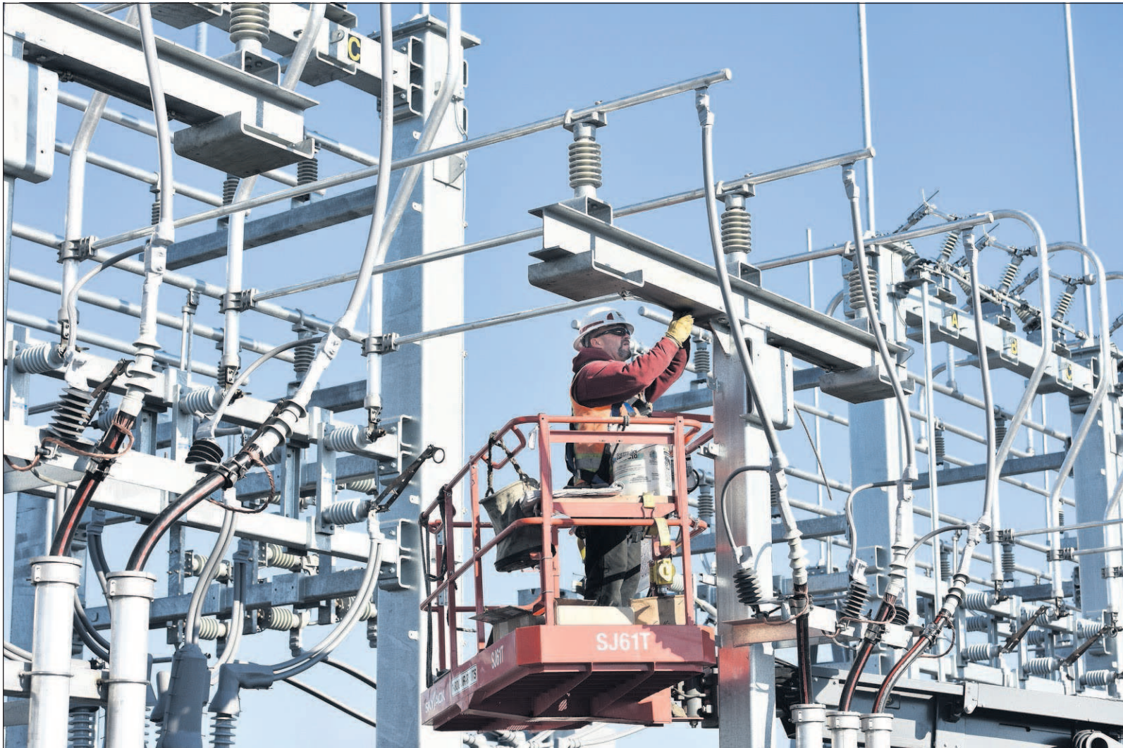
Staff photo by E.J. Harris Substation technician Darrin Balch with Potelco Inc. of Sumner, Washington, installs a ground wire on a riser structure at the new Umatilla Electric Cooperative substation off East Elm Avenue in Hermiston on Wednesday.
