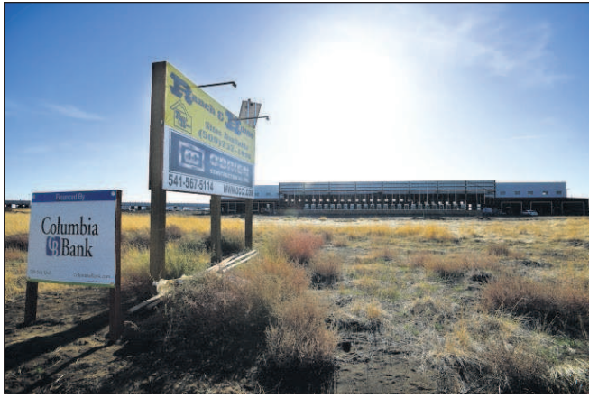
Construction continues on the new Ranch and Home site on Monday in Hermiston.
