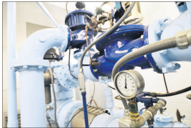
The water pressure for the city of Pendleton's well water system reads on a gauge at city well 14 on the west side of Pendleton. The city currently operates eight wells for its drinking water system. Staff photo by E.J. Harris
