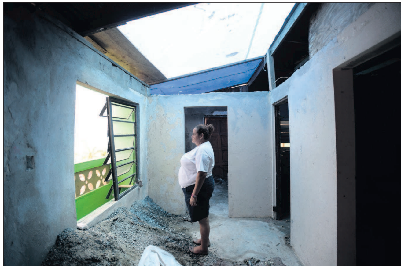
La Perla resident Maritza Rosado stands inside her roofless home after Hurricane Maria, in San Juan, Puerto Rico, Monday. The island territory of more than 3 million U.S. citizens is reeling in the devastating wake of Hurricane Maria.
