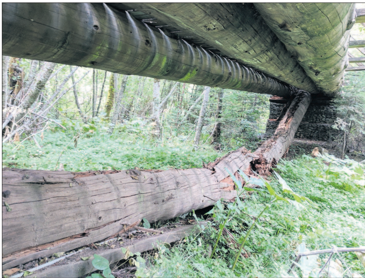
Some structural supports have collapsed beneath the Burnt Cabin Bridge, located six miles up the South Fork Walla Walla Trail. The bridge is closed until further notice.
