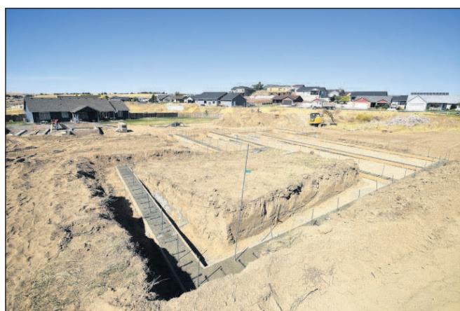
Staff photo by E.J. Harris The concrete foundation for a new home sets in the afternoon sun Tuesday in the Sunridge Estates housing development in Pendleton.
