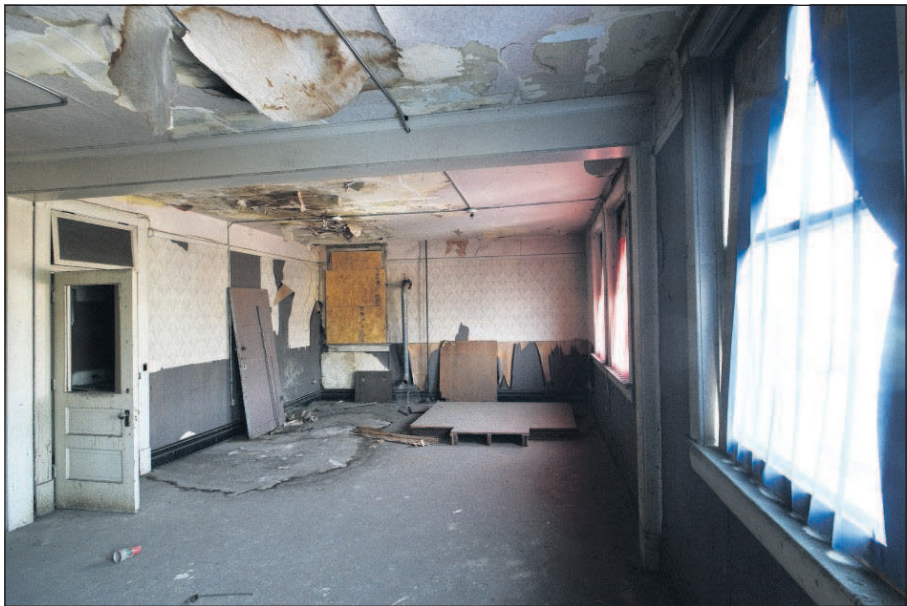
Water stains and other damage in a room on the second floor of the Woodmen of the World building on Southeast Court Avenue in Pendleton.
