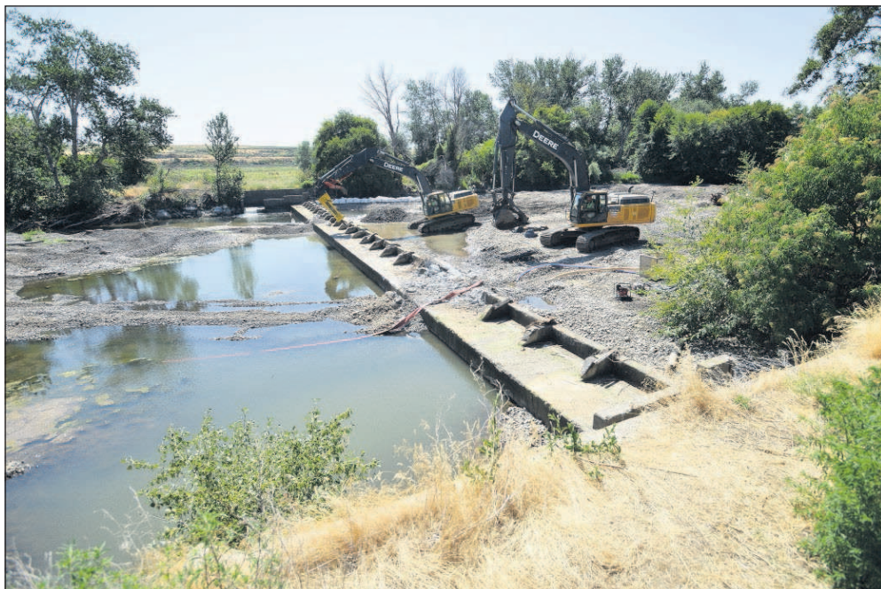
A pair of excavators work on removing the 100-year-old Dillon Dam on Wednesday near Echo.
