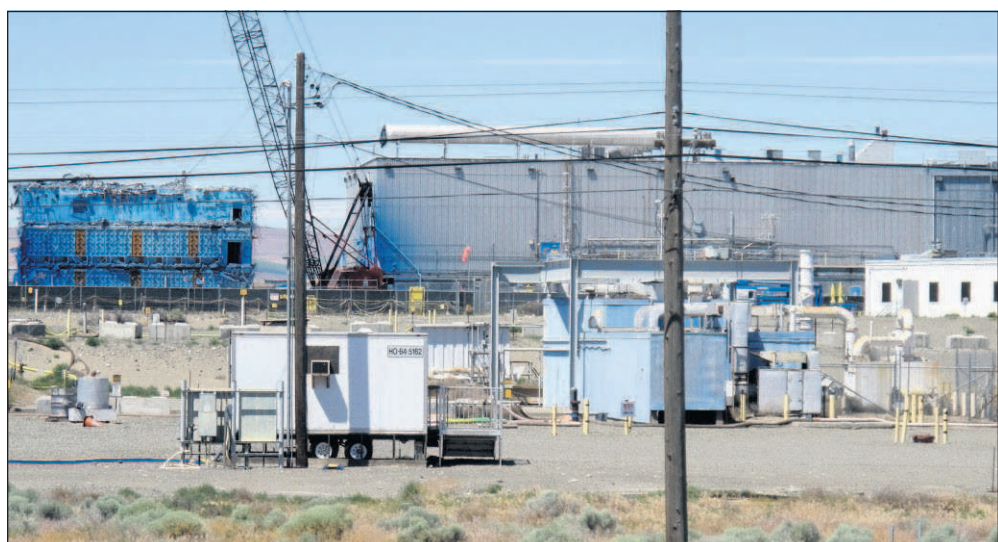
In this June 13 photo, demolition work continues on the Plutonium Finishing Plant on the Hanford Nuclear Reservation near Richland, Wash. The U.S. Department of Energy says there is a high risk that a second tunnel filled with radioactive waste might collapse on the Hanford site. A tunnel partially collapsed at the site on May 9 forcing some 3,000 workers to seek shelter for a few hours.
