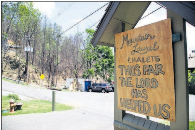
In this May 20 photo, a handmade sign stands in front of the fire-damaged Mountain Laurel Chalets.
