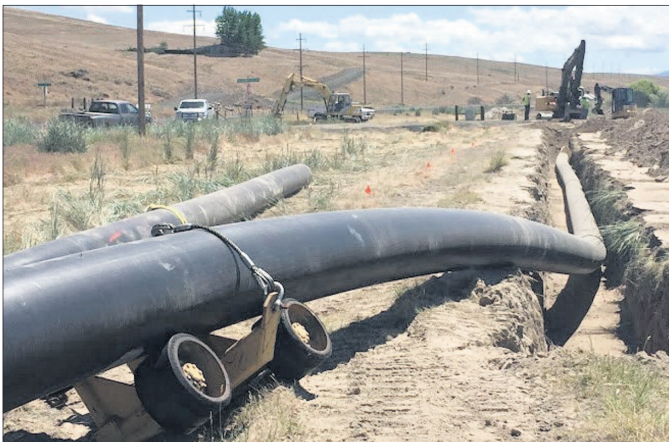
Construction is underway on the Heppner-Lexington Diversion Pipeline, which will carry supplemental irrigation water from Willow Creek Reservoir.
