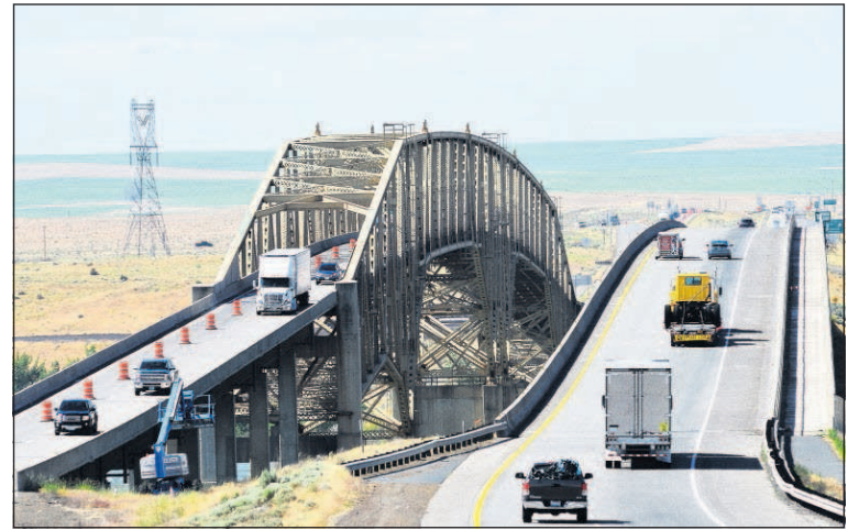
Staff photo by E.J. Harris South bound traffic is reduced to one lane at the Umatilla bridge over the Columbia River on Monday in Umatilla.
