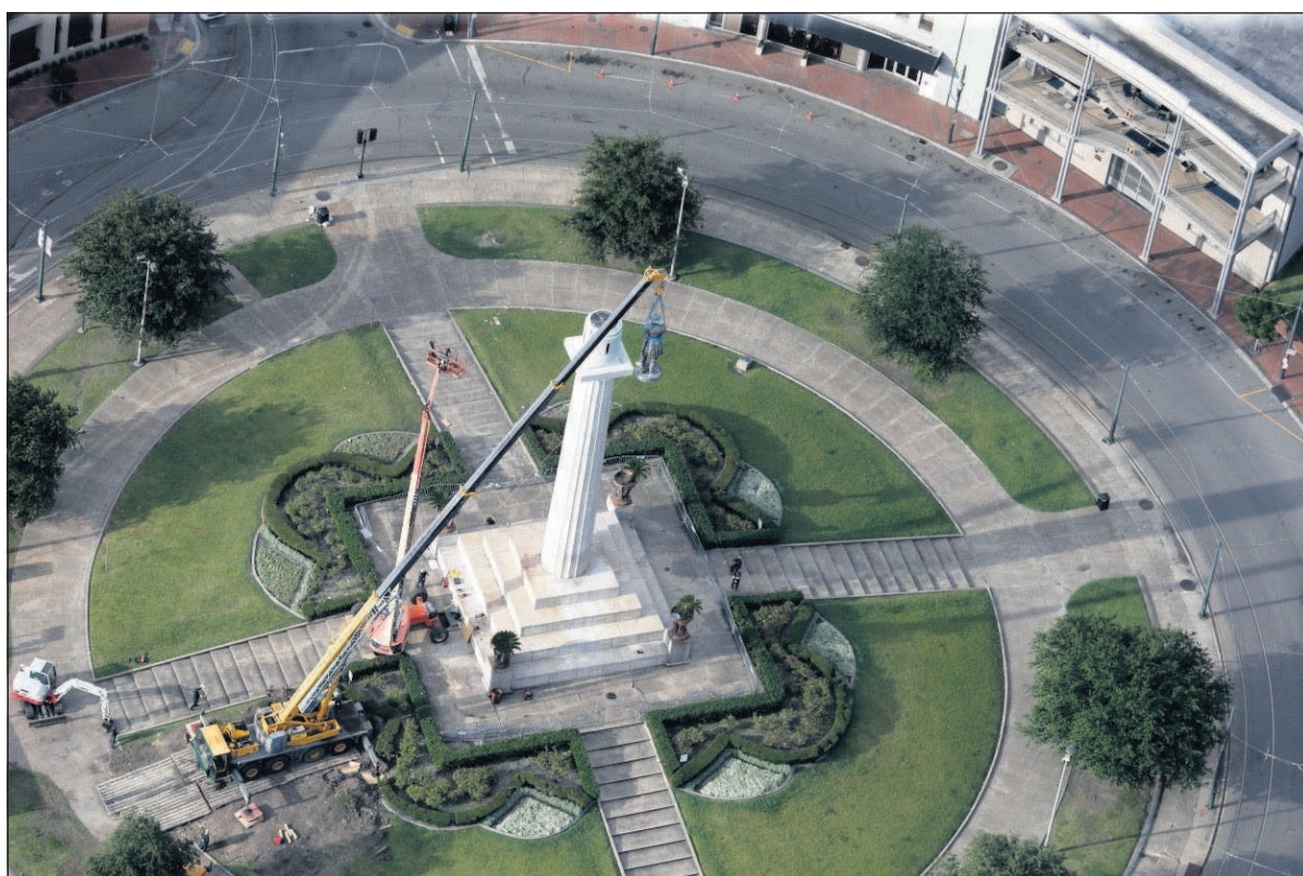
Workers take down the statue of former confederate general Robert E. Lee, which stands over 100 feet tall, in Lee Circle in New Orleans on Friday.
