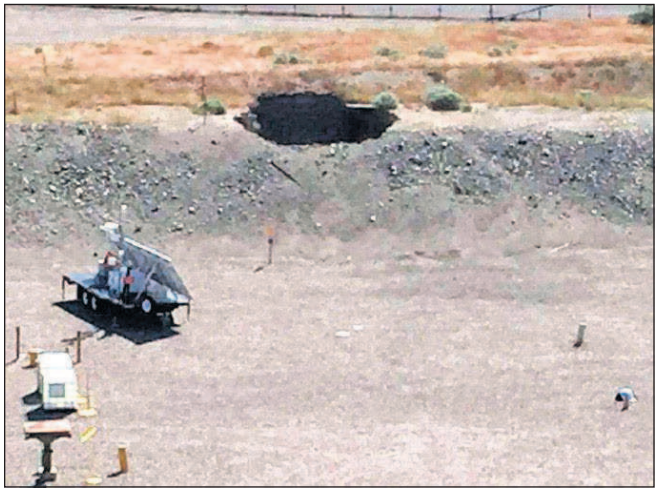
This image provided by the U.S. Department of Energy shows a 20-foot by 20-foot hole in the roof of a storage tunnel at the Hanford Nuclear Reservation Tuesday.
