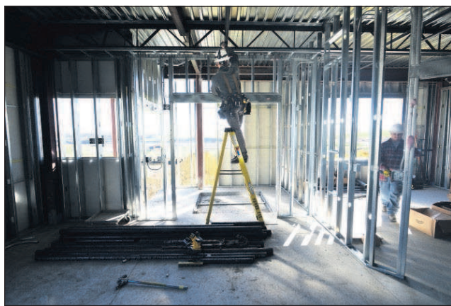
Construction continues on the FARM (Facility for Agricultural Resource Management) building Monday on the BMCC campus in Pendleton.
