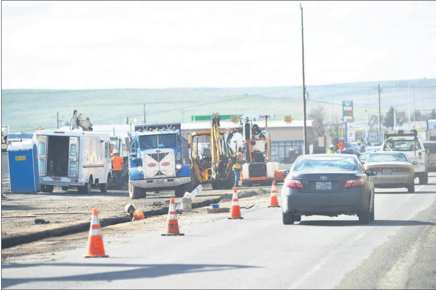
Traffic passes a construction zone Monday on Westgate in Pendleton. The construction zone is blocking one lane as crews dig a trench to replace a section of the water main.
