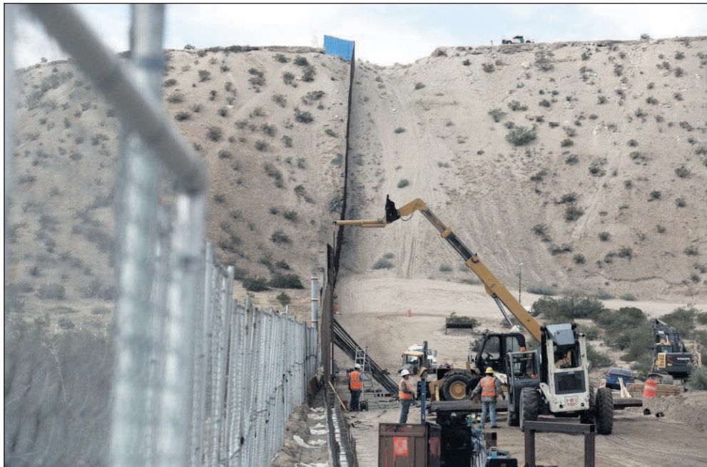
In this Nov. 10, 2016 file photo, workers continue work raising a taller fence in the Mexico-US border area separating the towns of Anapra, Mexico and Sunland Park, N.M. U.S.
