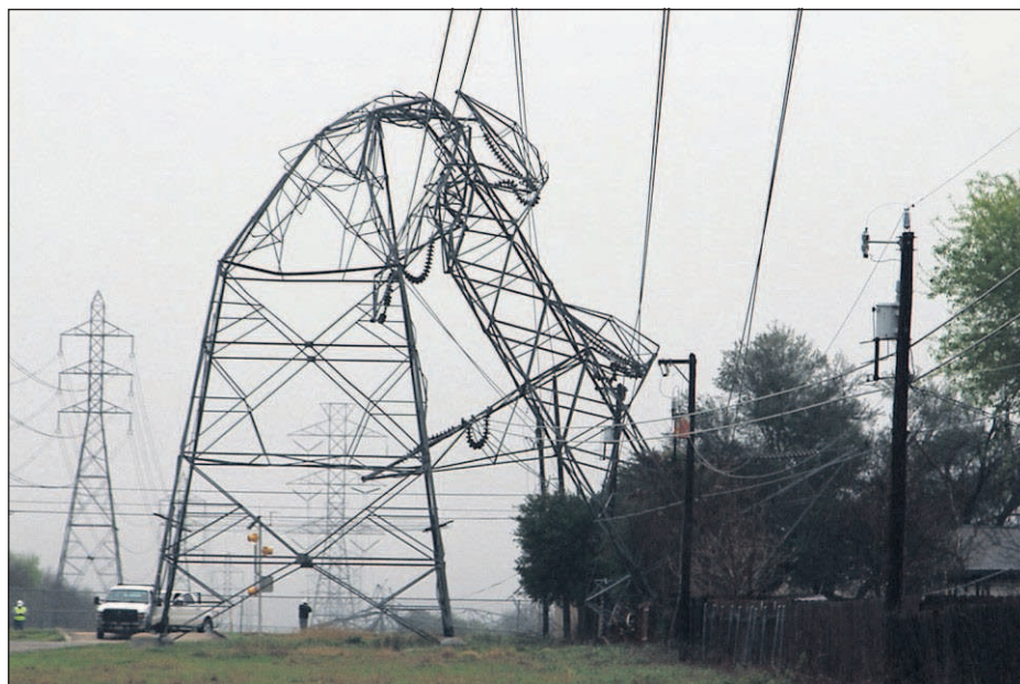
Tyler White/The San Antonio Express-News via AP A CPS Energy transmission tower is bent in half Monday in San Antonio. Severe storms pushed at least two tornadoes through parts of San Antonio overnight, ripping the roofs off homes and damaging dozens of other houses and apartments yet causing only minor injuries, authorities said Monday.
