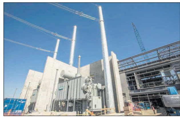
Contributed photo by Michael Durham Transformers surrounded by blast walls, which isolate individual transformers in case of failure, are shown during construction of the Carty Generating Station in August 2015.
