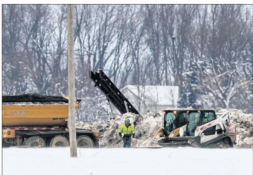
Crews work Thursday to clean up a diesel fuel spill after a pipeline owned by Magellan Midstream Partners broke on Wednesday. Chris Zoeller /Globe-Gazette via AP
