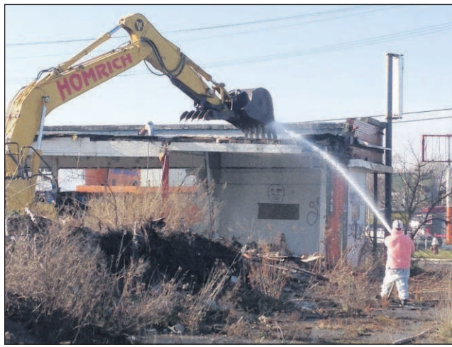
An excavation crew begins demolition of a vacant building on Detroit's west side Wednesday.
