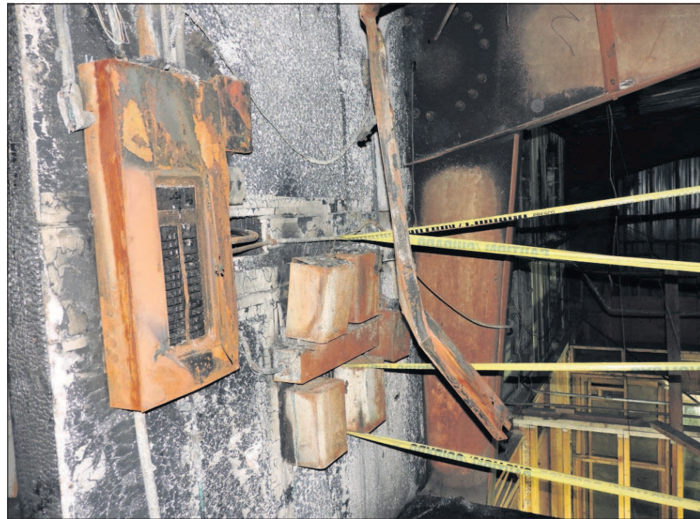
A power strip plugged into this wall is believed to have caused a June 20 fire at the Columbia Court Club.
