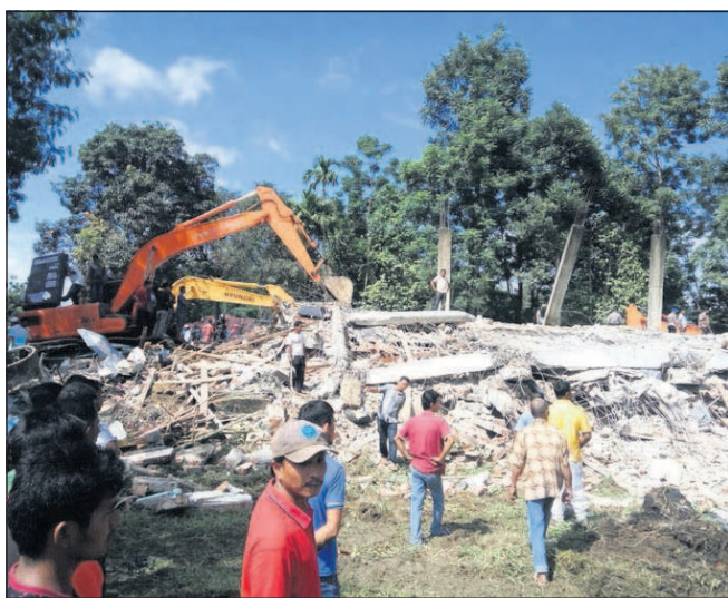
Rescuers use heavy machine to search for survivors under the rubble of a collapsed building after an earthquake in Aceh province, Indonesia, Wednesday. A strong undersea earthquake rocked Indonesia's Aceh province early on Wednesday, killing a number of people and causing dozens of buildings to collapse.
