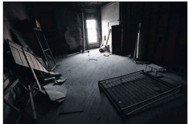
Staff photo by E.J. Harris Many of the upstairs apartments in the LaDow block have fallen into disrepair.
