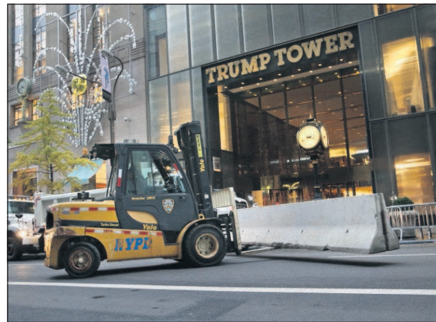
Police officers help install concrete barriers around Trump Tower, the home of President-elect Donald Trump, in New York, Wednesday.
