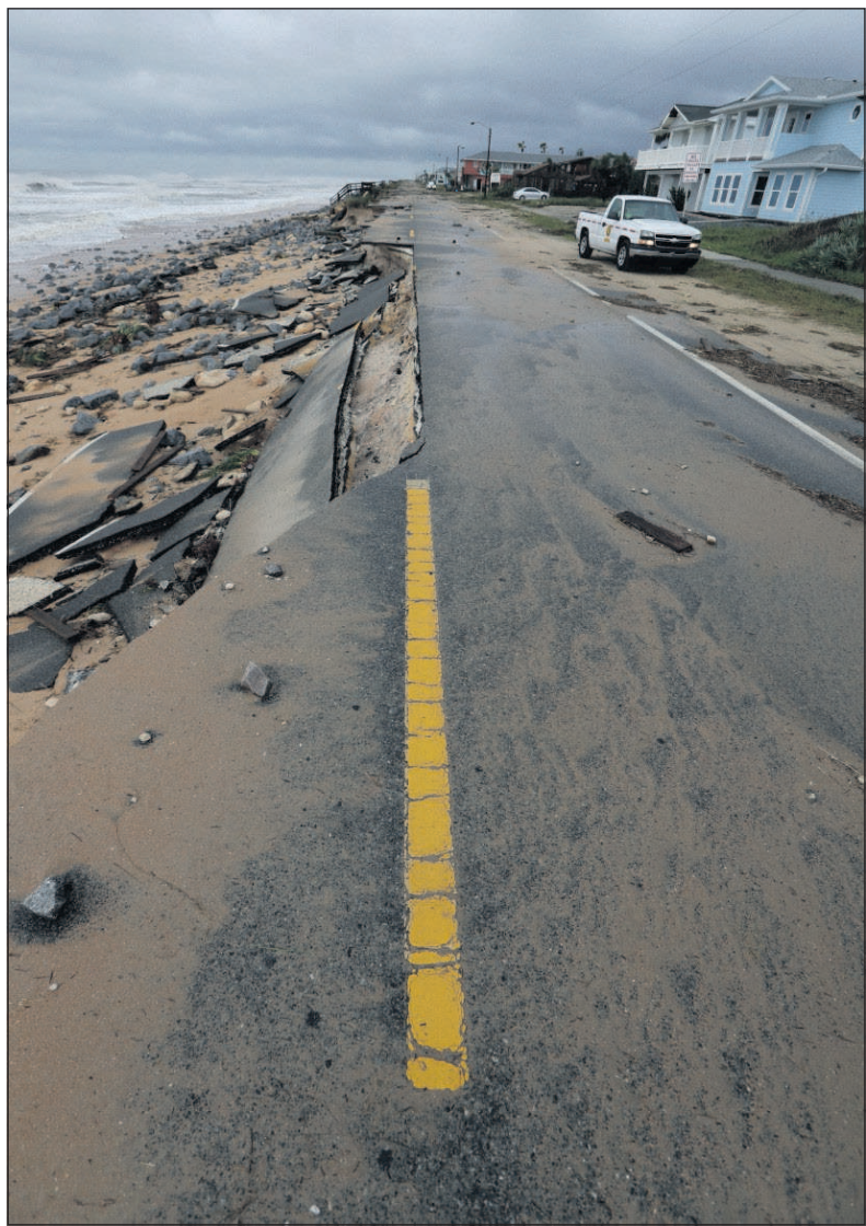
An official vehicle navigates debris as it passes along Highway A1A after it was partially washed away by Hurricane Matthew, Friday in Flagler Beach, Fla.
