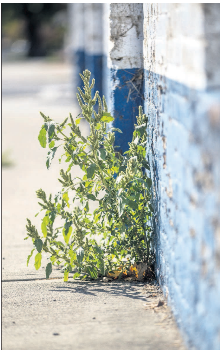
A weed grows from a crack at the base of the old Pendleton Grain Growers retail store in Athena.
