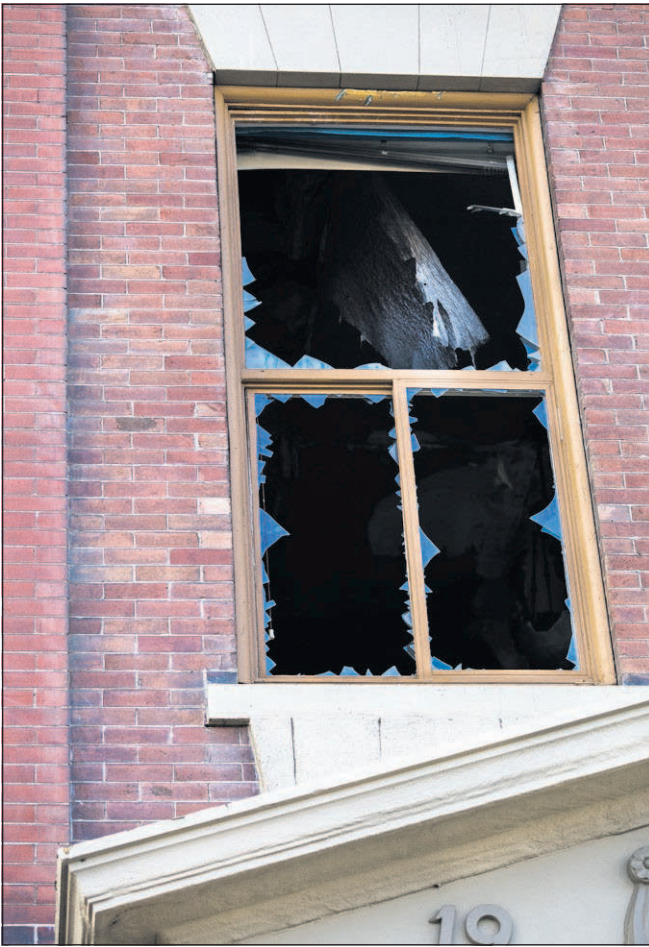
A charred curtain flaps in the breeze Wednesday in a second-story window of the Old City Hall, which has remained a burned-out shell since the 2015 fire that killed 25-year-old Eduard Quezada.
