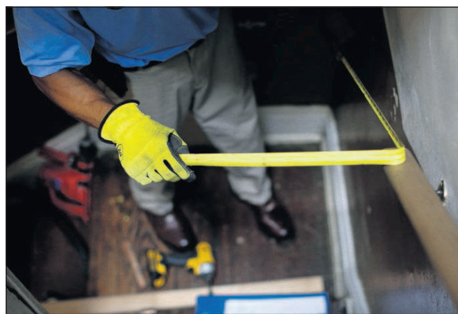
In this June 2013 file photo, a construction worker takes a measurement while installing a banister in a staircase in a home in Baltimore.
