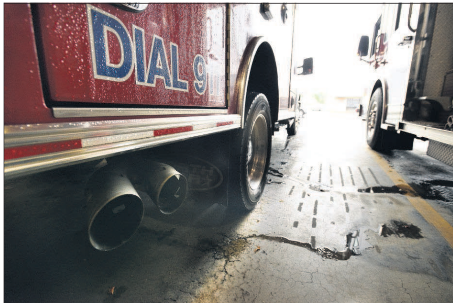
Residue from years of exhaust from diesel engines has coated many areas of the main fire station raising possible health concerns for firefighters. Diesel exhaust is a known carcinogen.
