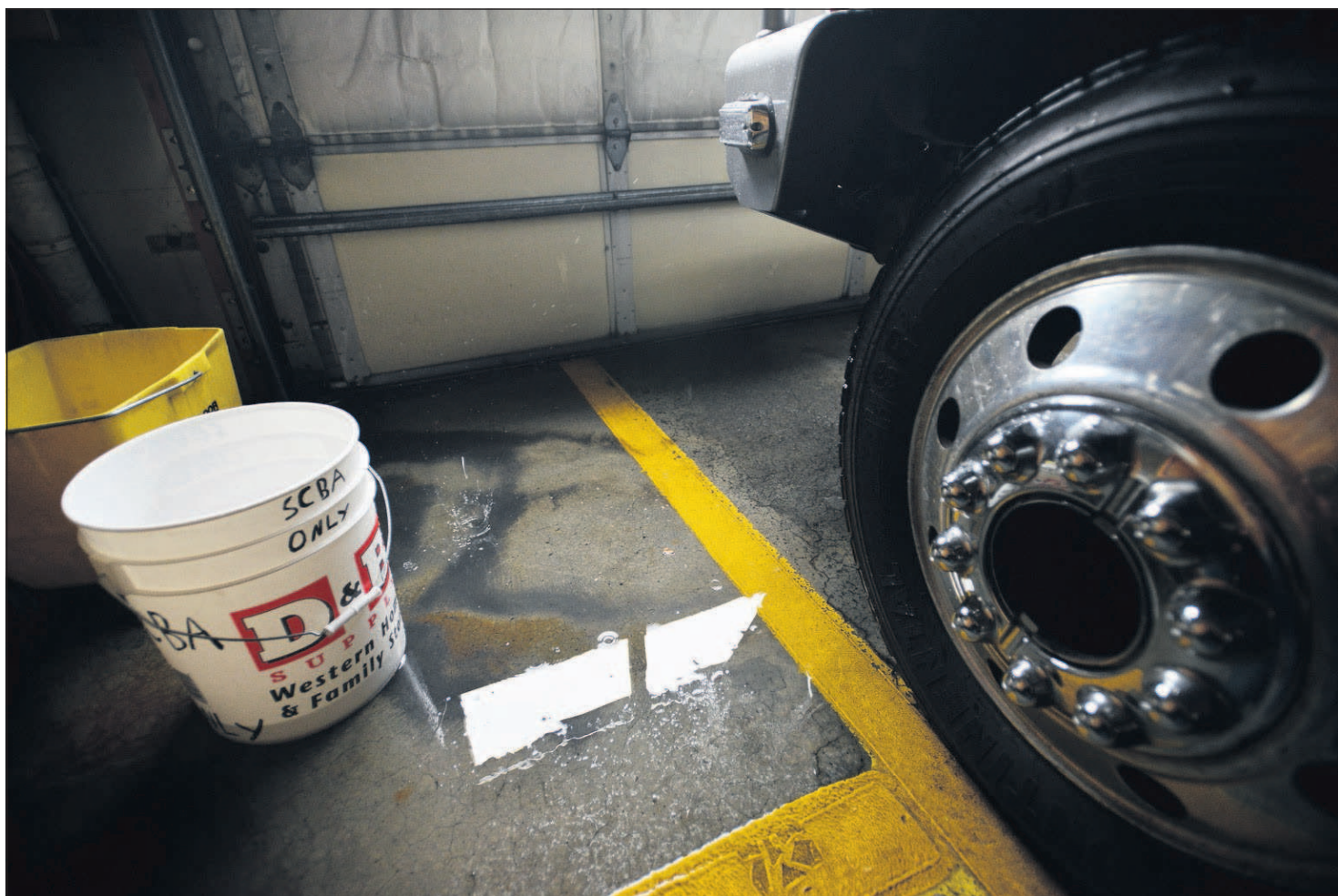
Water from recent rainfall leaks through the roof of the main fire station and falls into buckets and on the ground Monday at the main fire station in Pendleton. Staff photo by E.J. Harris
