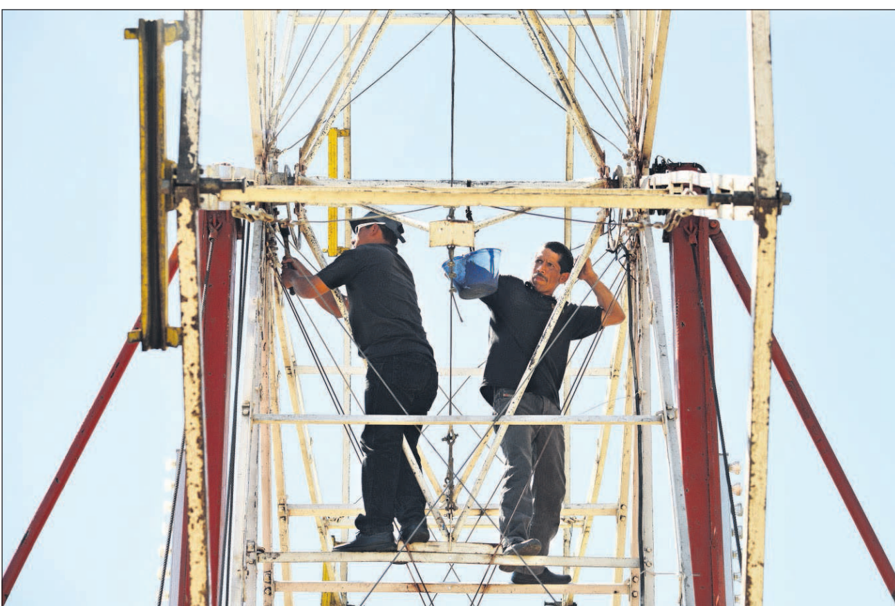
Carnival workers assemble the Ferris wheel on Thursday at the Umatilla County Fair in Hermiston.
