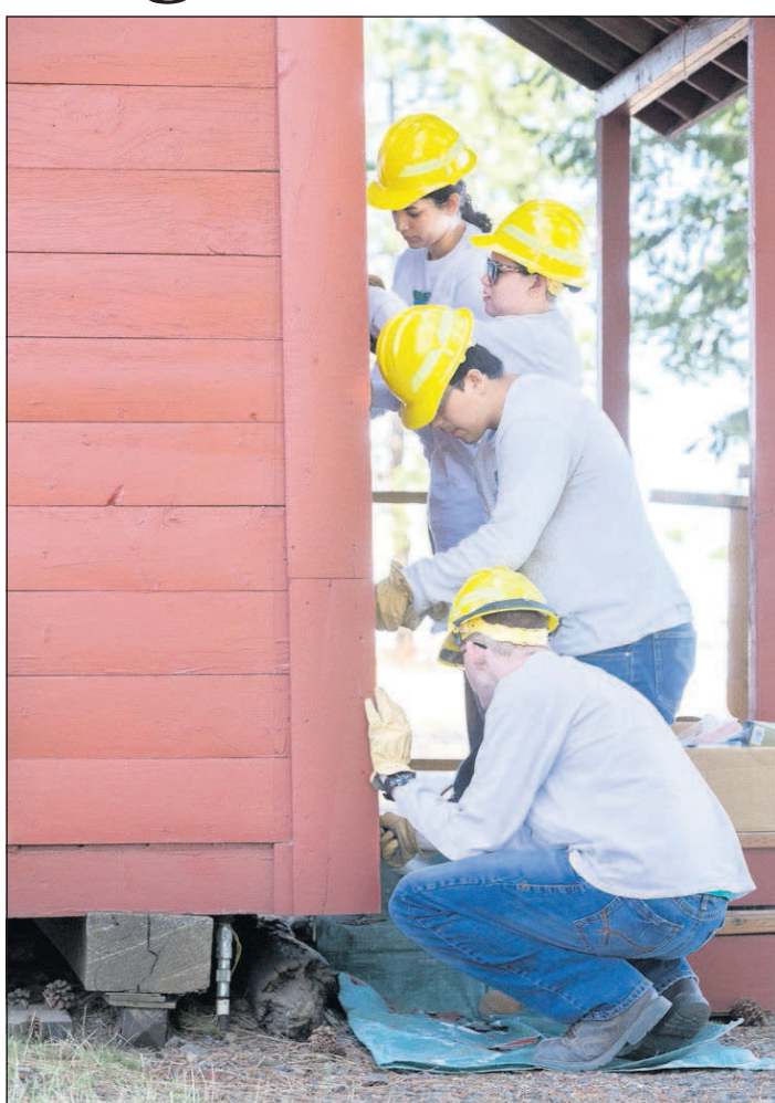
Raeana Mikel, Angela Heay, Trevor Magers and Nathan Van Dusen scrape the sides of the Summit Cabin on Thursday as one of their projects for the Oregon Youth Conservation Corp. The rustic Forest Service guard station, located in the Blue Mountains, was built in 1938 and used as a cookhouse for fire crew tent camps in the 1970s.
