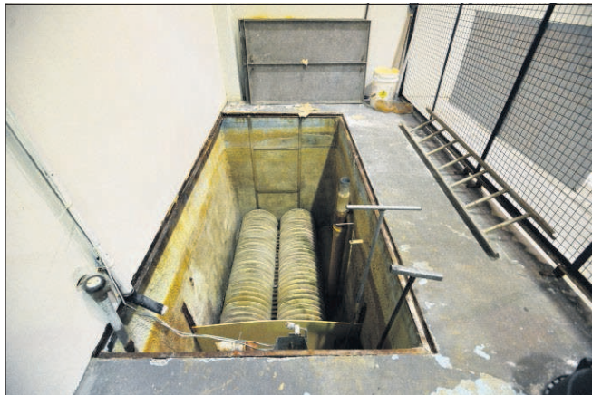
A section of the pool's water filtration system at BMCC in Pendleton.
