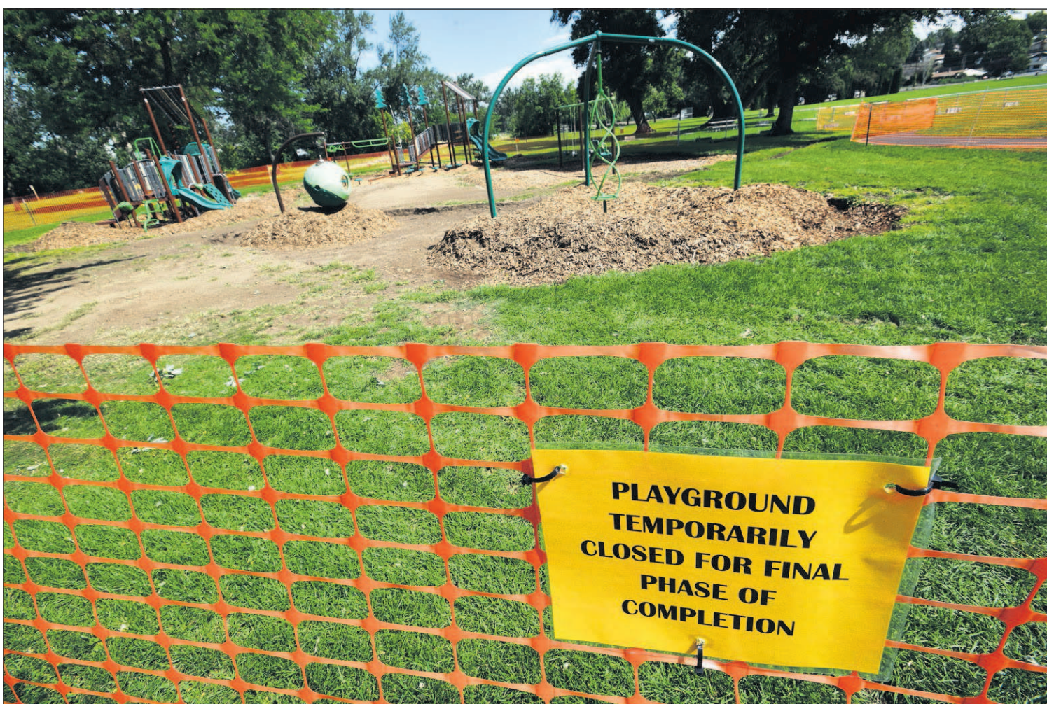
Orange fencing surrounds a play area that is under construction at Community Park in Pendleton.
