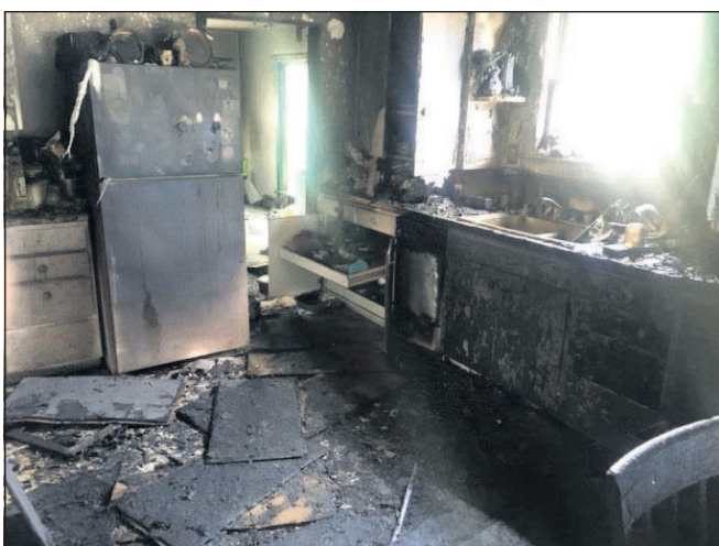
Contributed photo by Ricardo Lara Extensive damage to a house on West Crockett Lane in Milton-Freewater can be seen after the home caught fire Monday night. An official cause is yet to be determined but residents suspect fireworks.
