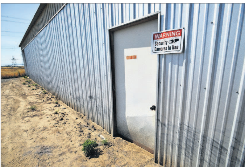
The Linds continue to have problems with burglars. Last week someone attempted to kick in this door to a storage building at the Lind's home, according to Bernard Lind.
