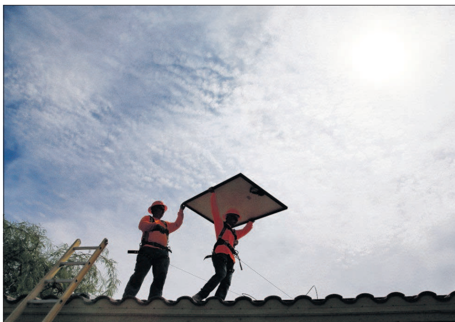
Electricians install solar panels on a roof for Arizona Public Service company in Goodyear, Ariz.
