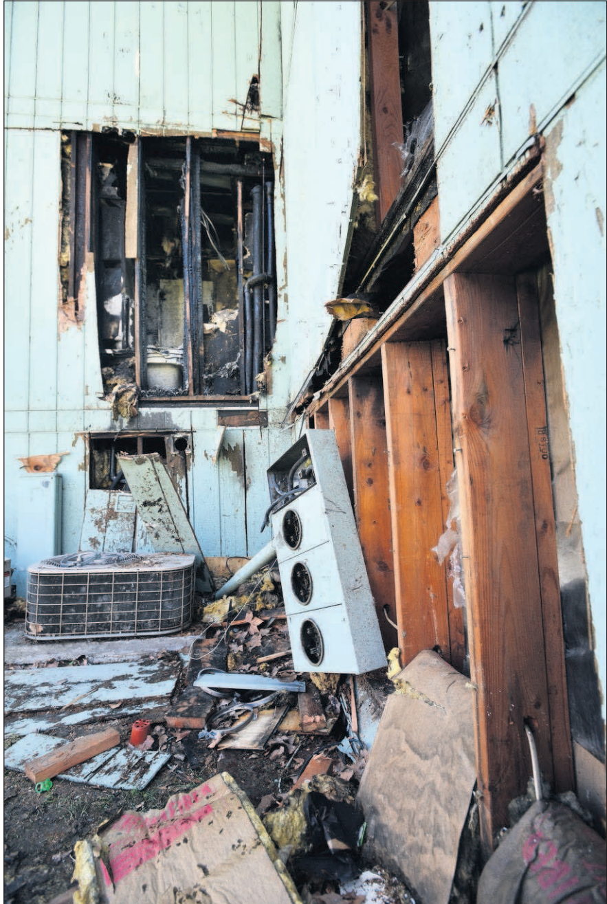
Holes are tom out of the walls of a building at the Marina Apartments where firefighters were attempting to find and extinguish the slow moving fire.
