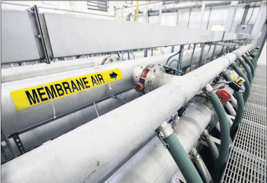
The membrane train is the central hub of the Pendleton water treatment plant with it’s more than 3,000 miles of micro-porous membrane that filters the water.
