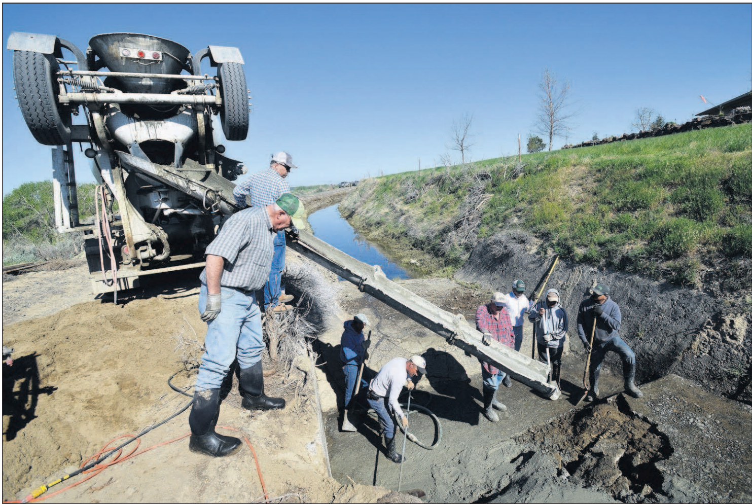
Staff photo by E.J. Harris Workers with the Stanfield Irrigation District work on patching a ruptured spillway on Thursday in one of their irrigation canals near Echo.
