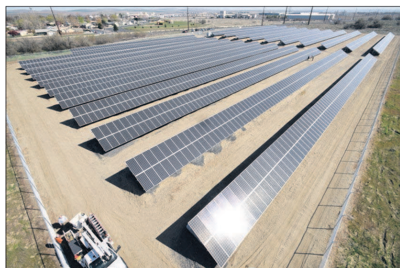
The Umatilla Electric Cooperative now has the largest consumer-owned solar project in the state with their 1.3 megawatt solar array outside of Umatilla.
