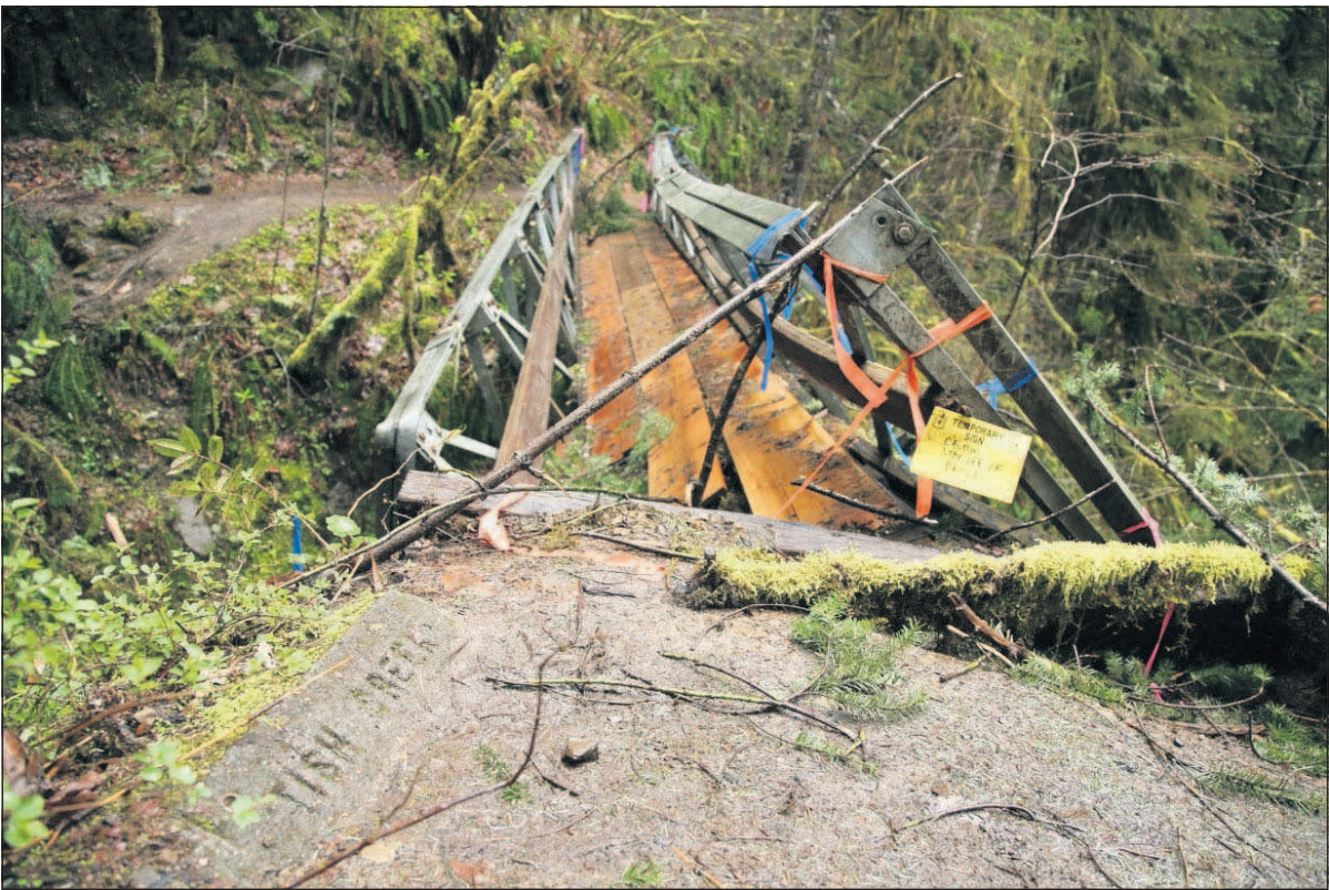
In this March 22 photo, the bridge over Tish Creek on the popular Eagle Creek Trail in the Columbia River Gorge was destroyed by a fallen tree in December 2015. Officials with the U.S. Forest Service estimated it would take at least a year to replace it. Winter can be a tricky season in the Columbia River Gorge. High rainfall leads to gushing waterfalls, but it also leads to crumbling earth.
