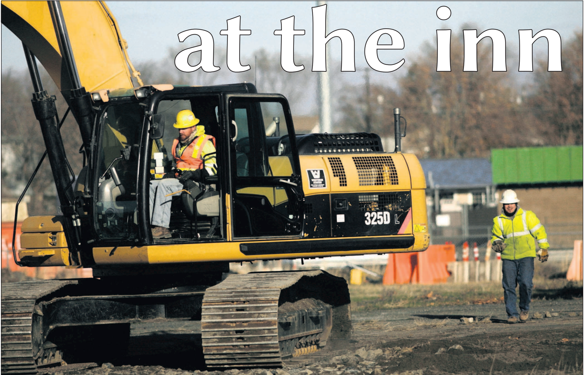
Site preparation work has started at the location where a four-story Holiday Inn Express will be build at the corner of West Hermiston Avenue and Highway 395. Heavy equipment operators were working on the site Tuesday, Dec. 15. According to Mark Morgan, assistant city manager for Hermiston, building permits were purchased for the location last week.
