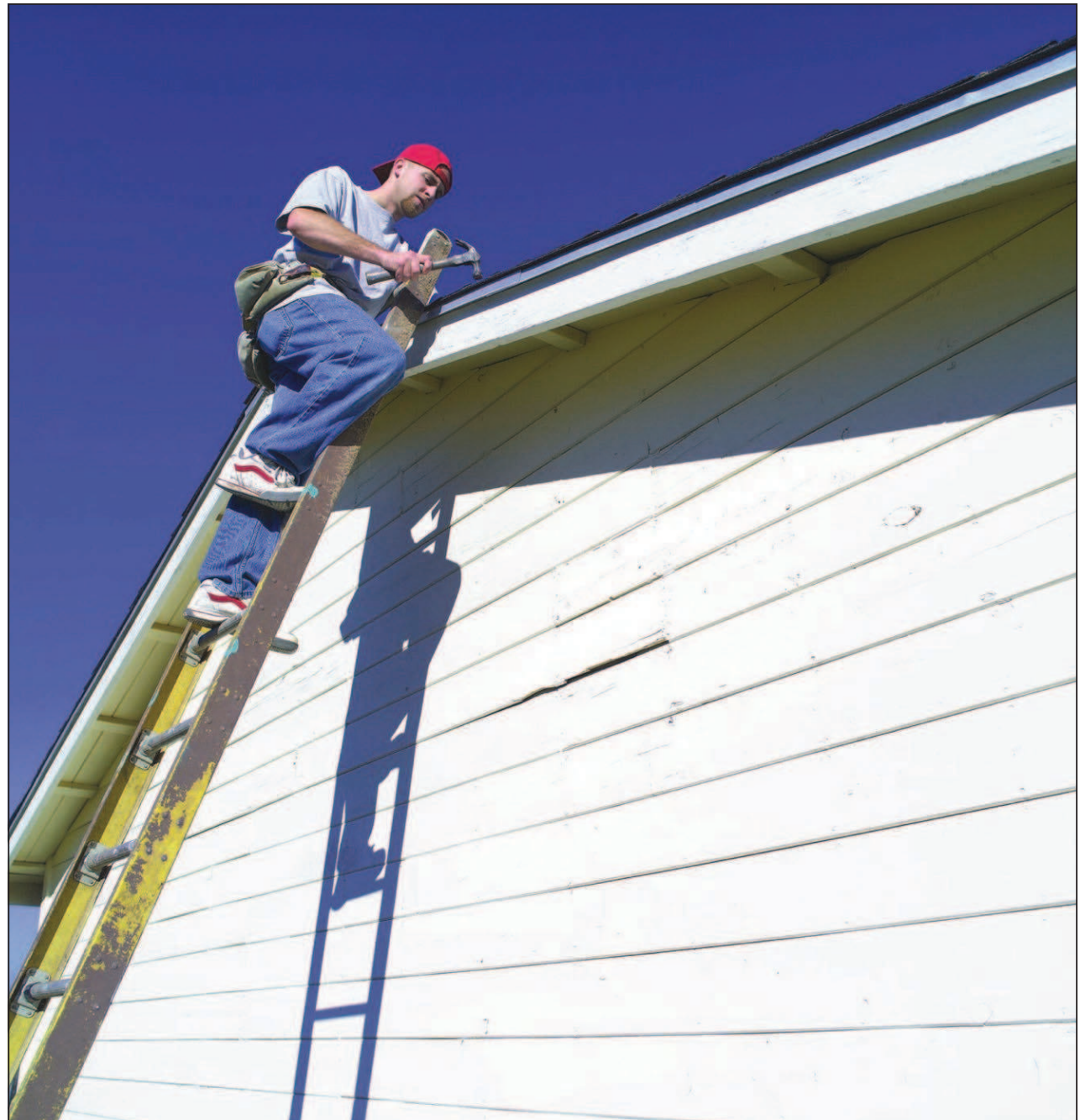
Home buyers may be able to negotiate that the sellers repair major structural issues, such as a leaky roof. If not, negotiate a lower sale price.
