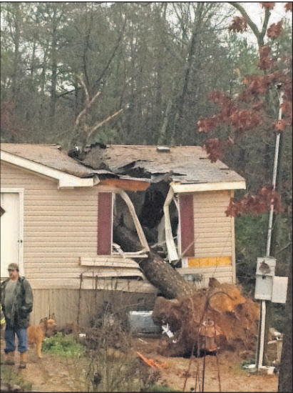
Pope County Sheriff's Department photo via AP This photo provided by the Pope County Sheriff's Department shows a storm damaged home outside of Atkins, Ark., on Dec. 23.
