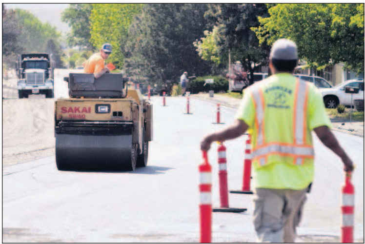
A new layer of asphalt is applied to Southwest Nye Avenue early last summer in Pendleton. EO file photo
