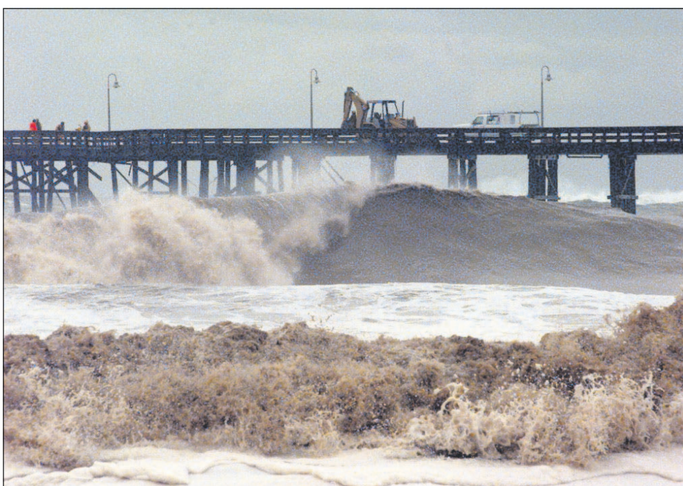
In this Feb. 2, 1998 file photo, work crews attempt to repair a damaged pier caused by waves that reached 15 feet from the massive El Nino-driven storm in Ventura, Calif.
