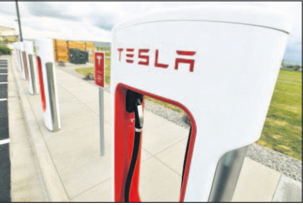
A Tesla supercharger was installed at the Arrowhead gas station in Mission earlier this year.
